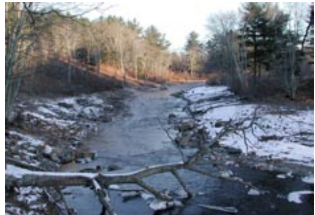
Sennebec Dam, in Union, Maine, before and after removal. Credit: John Catena, NOAA
